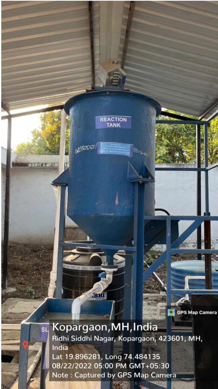
Effluent Treatment Plant
