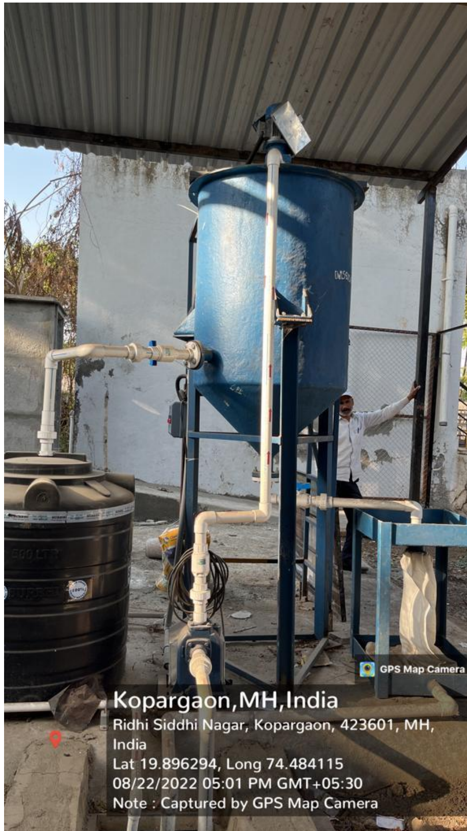
Effluent Treatment Plant
