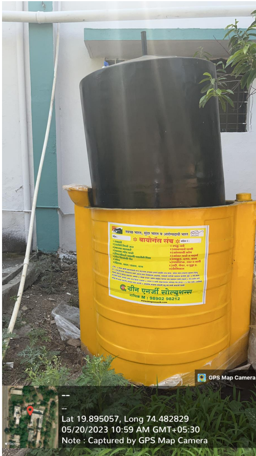
Biogas Plant at Ladies Hostel
