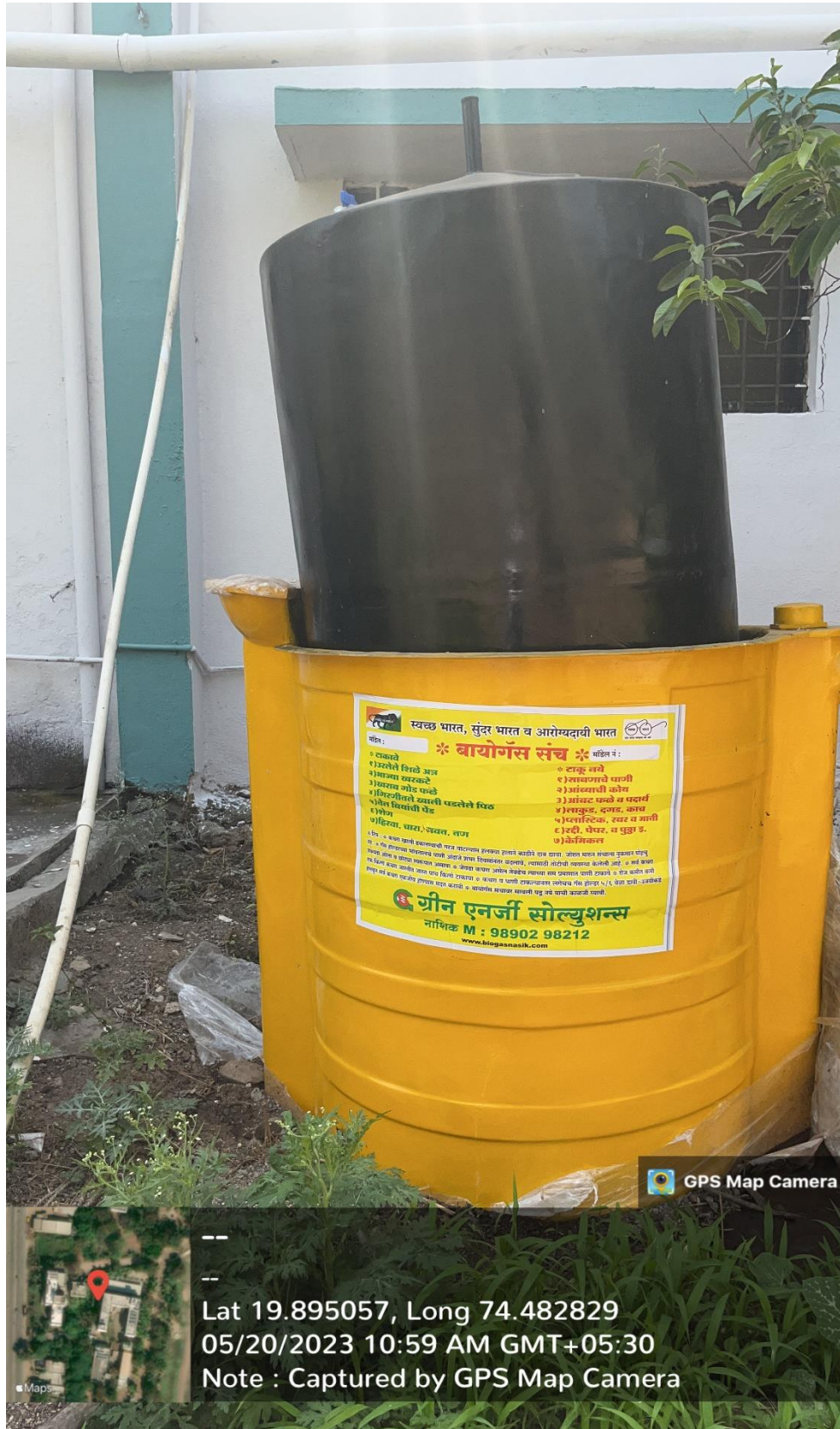
Bio Gas Plant at Girls Hostel
