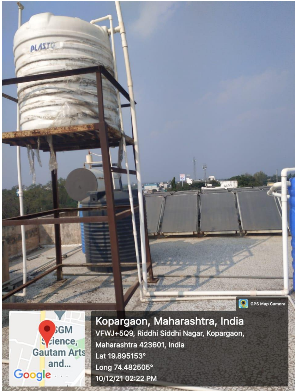
Solar Water Heaters at Hostel
