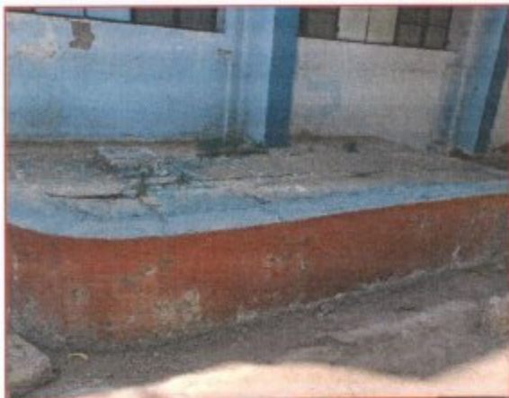
1. Drainage system of Hostel
