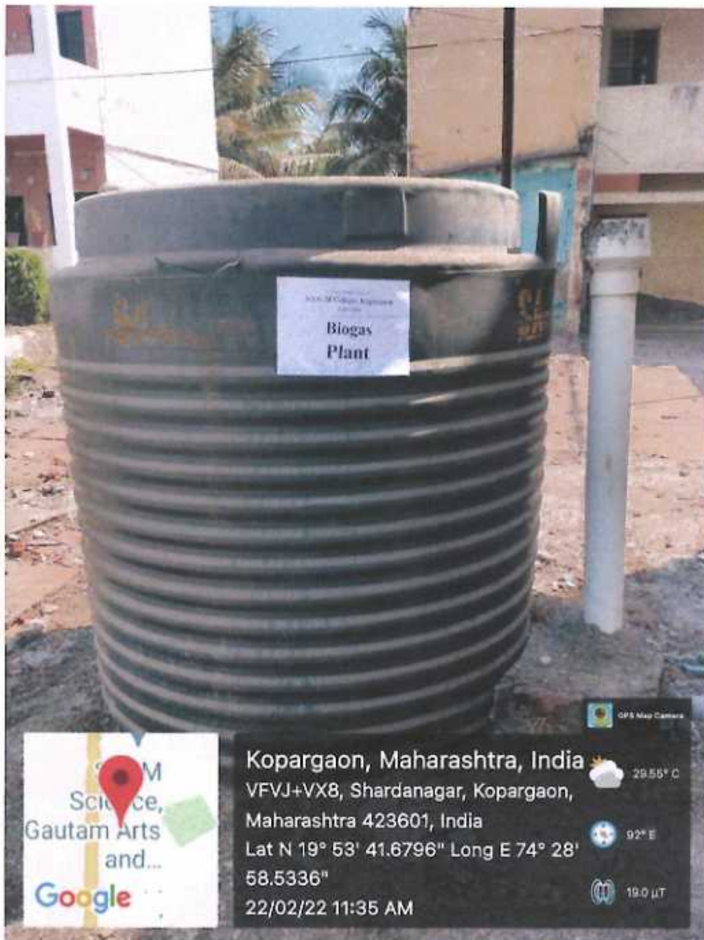
Biogas Plant at Ladies Hostel
