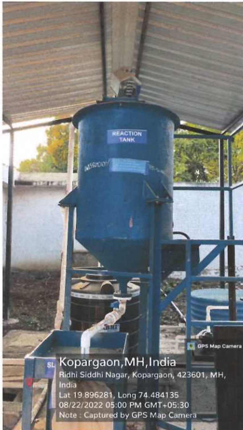
Effluent Treatment Plant
