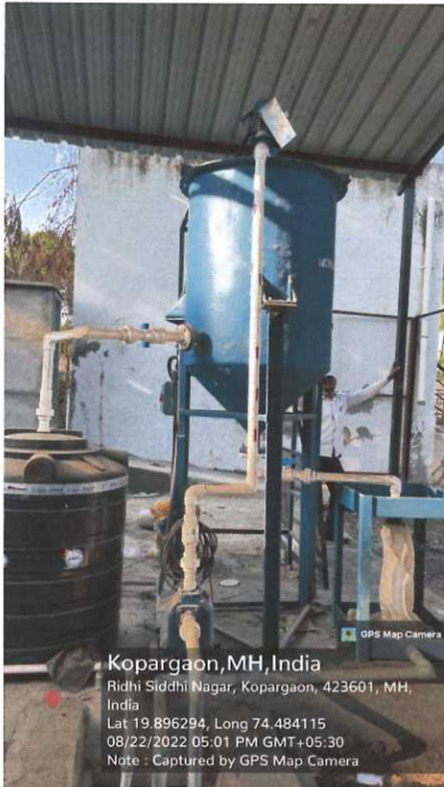
Effluent Treatment Plant
