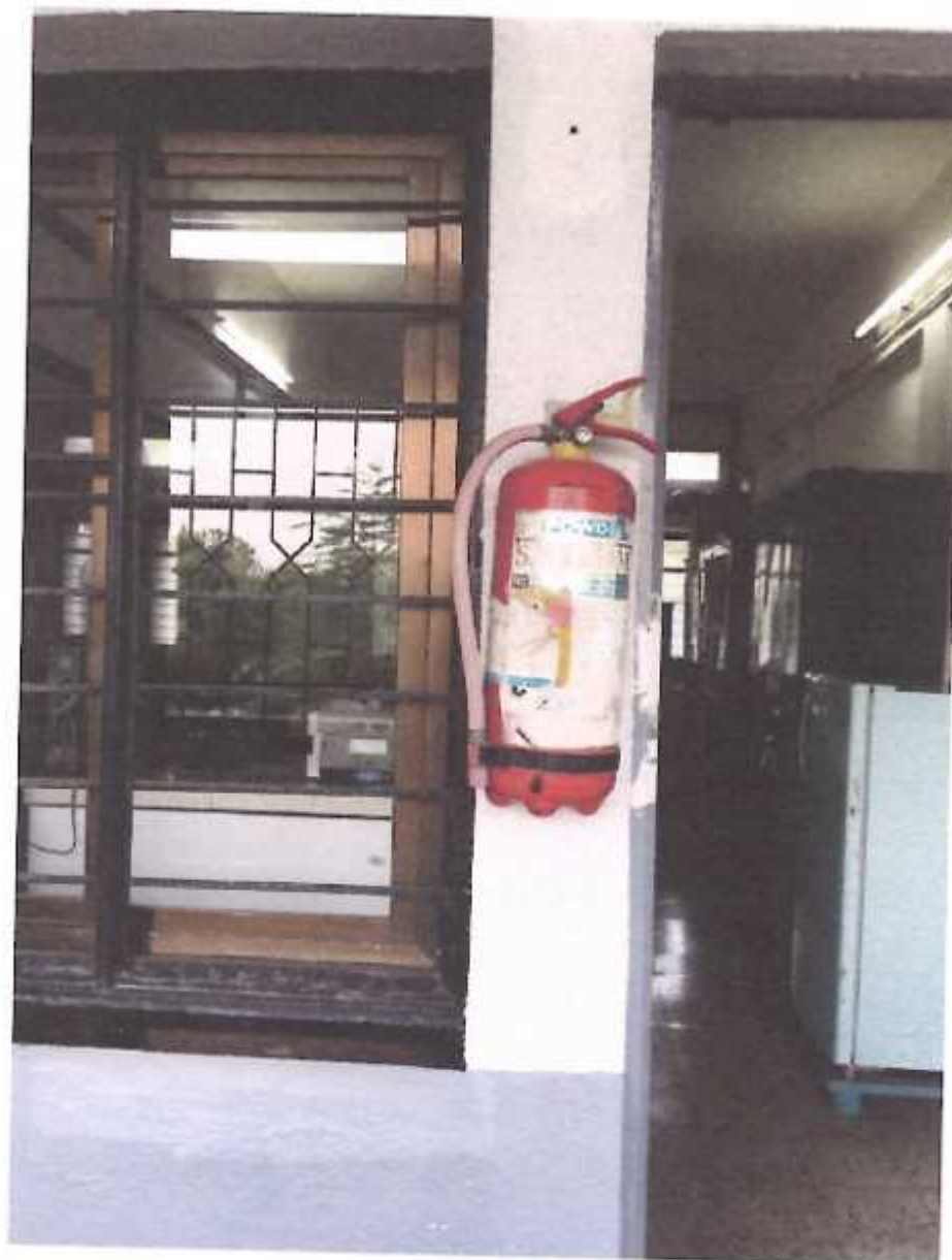
Fire Extinguishers at various places
