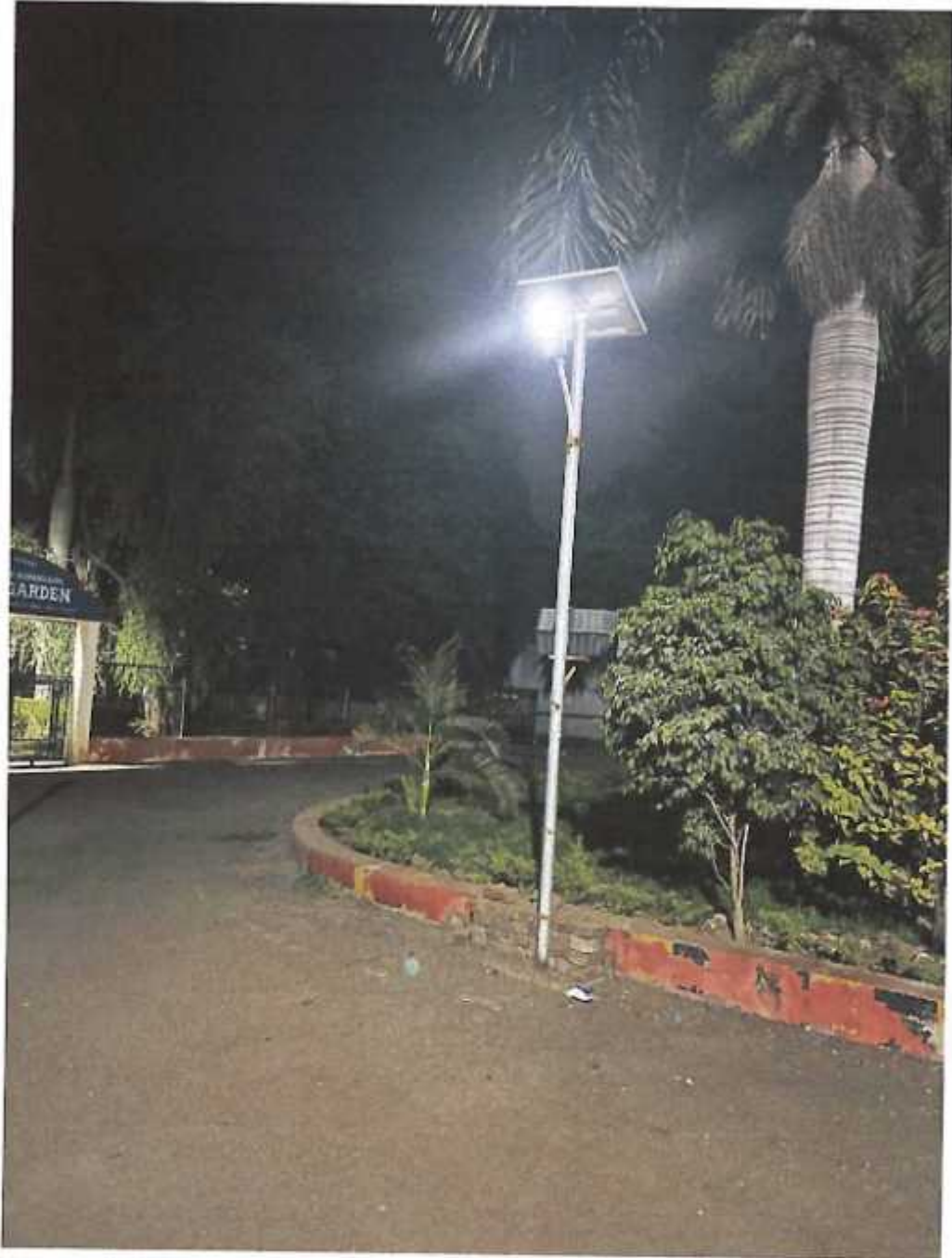
Sensor Based Solar Lights
