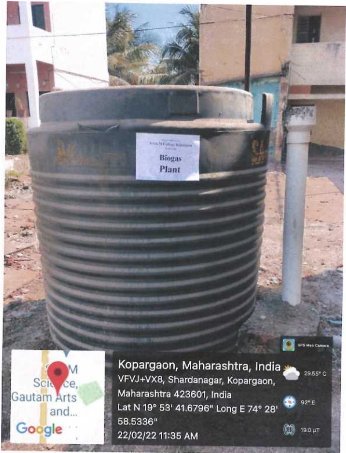
Biogas Plant at Girls Hostel
