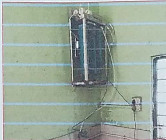
2. RO system in Hostel
