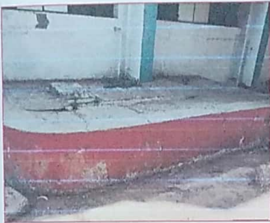
1. Drainage system of Hostel
