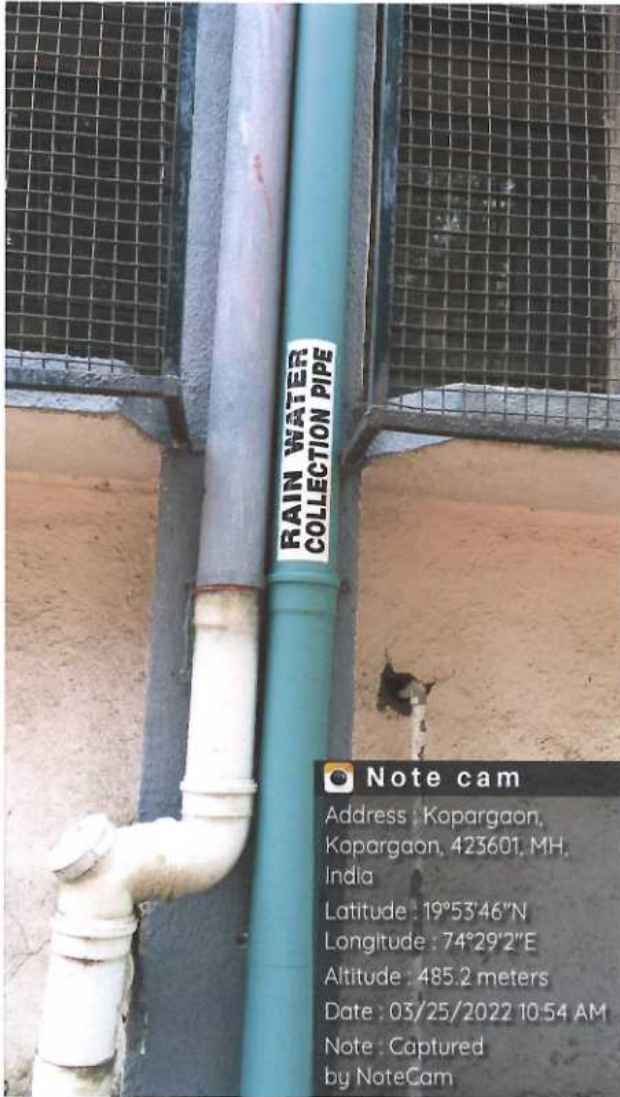
Rain Water Collection from Roof-top
